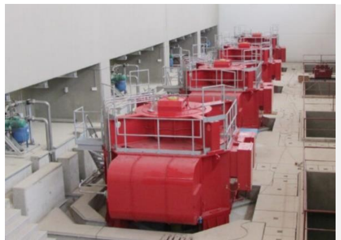
Figure 2. 4x12.1 MVA hydro generators manufactured by Gamesa Electric
